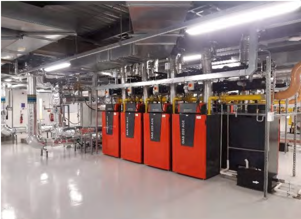
Figure 5 - Replacement Boilers at QMH, Dunfermline
