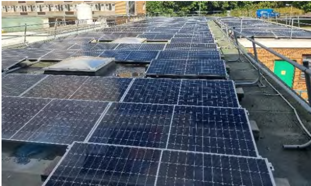
Figure 6 - Photovoltaics at VHK, Kirkcaldy
